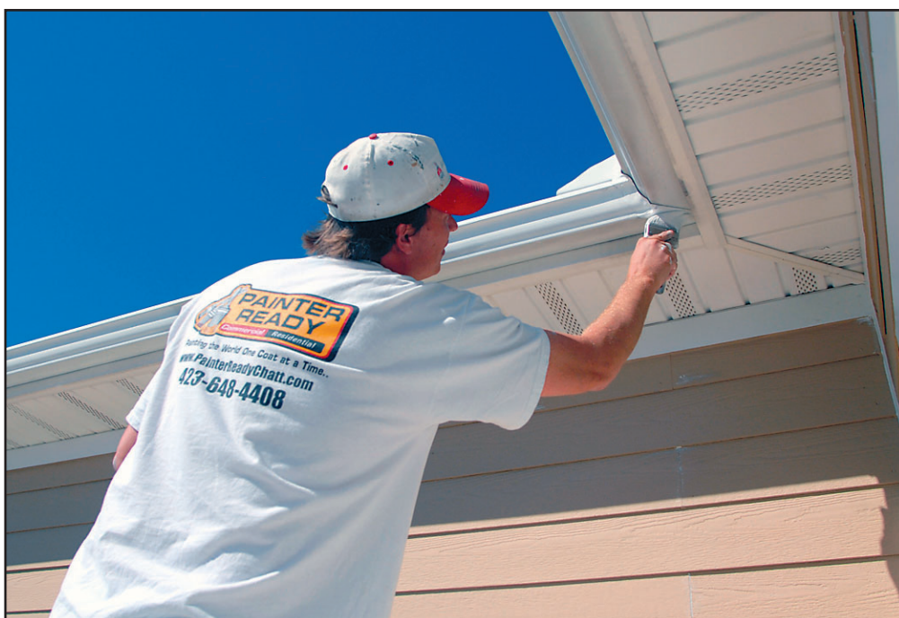
STAFF PHOTO BY LESLEY ONSTOTT Painter Ready employee Joe Shadwick paints the gutter of a house off Shallowford Road.
